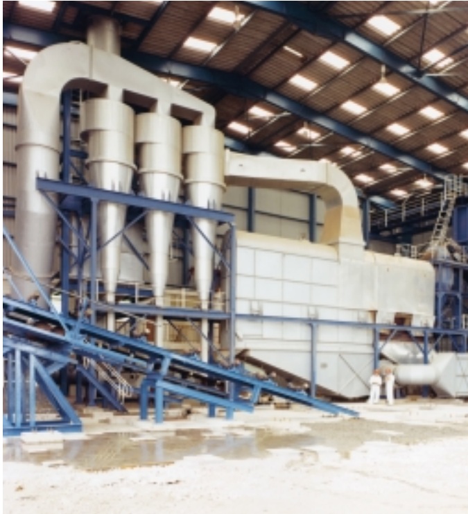
Combined fluid bed dryer/cooler for minerals
